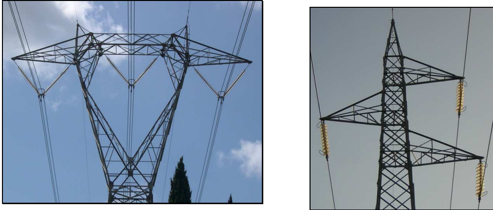
Figure 11 – Standard pylon head for a 380 kV power line (on the left) and for a 132 kV one (on the right)
